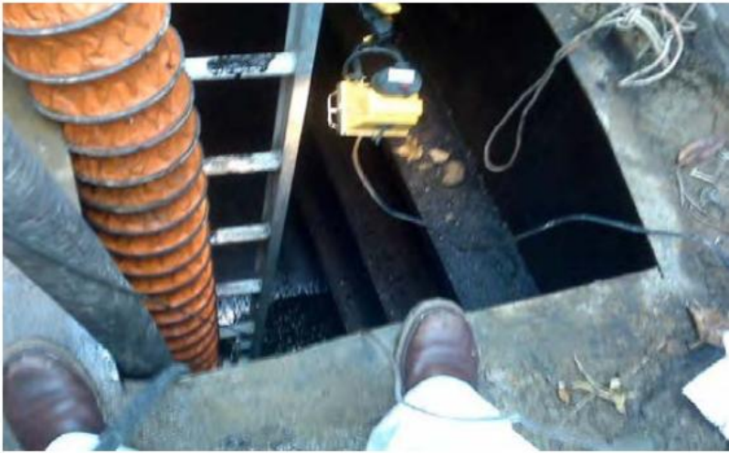
Ventilation hoses provide air and exhaust toxic vapors during confined space entry. A guardrail would also be necessary to protect workers from potential falls.
