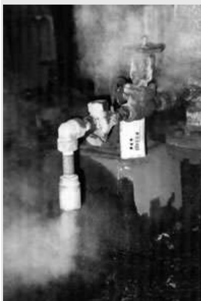
Typical steam discharge with silencer
